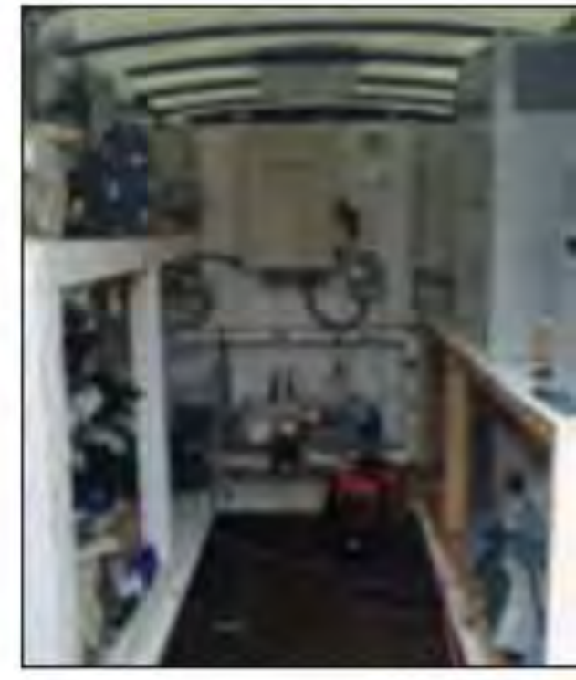
THE TRAILER CONTAINS TWO SEPARATE SYSTEMS, ONE FOR LARGE POOLS, THE OTHER FOR SMALLER BODIES OF WATER. BOTH INCLUDE OZONE, UV AND CHLORINE INJECTION, ALL OF WHICH CAN BE RUN SEPARATELY, IN TANDEM OR ALL TOGETHER.
